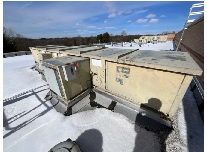
22 - ROOFTOP PACKAGED UNIT
