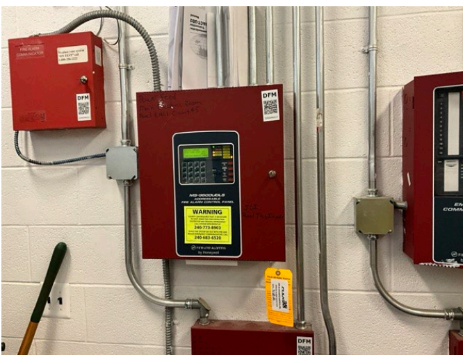
17 - FIRE ALARM PANEL
